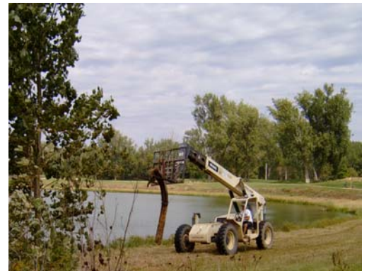
Mike Wallace drives the fork lift with a 20 foot section of rail to the Silver Hawks Ski Club area
